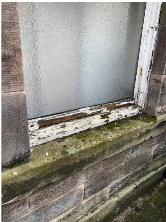
Figure 1 Sash window with decaying cill and bottom rail
